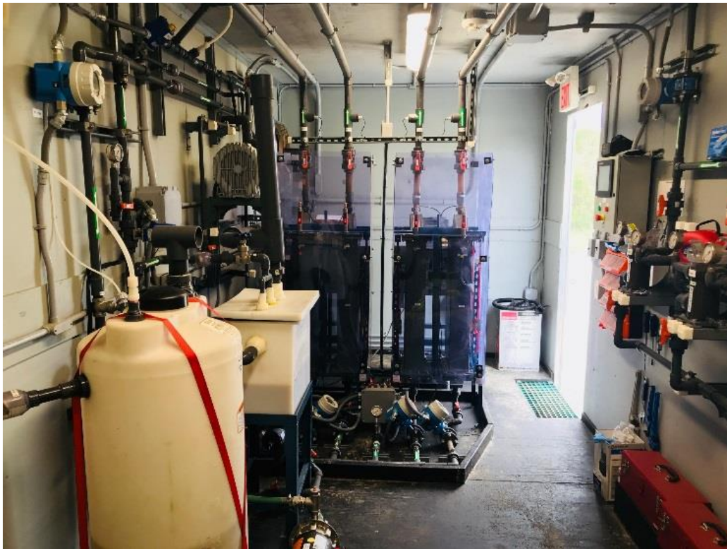
The Xogen AEO Treatment System, turnkey and fully automated
